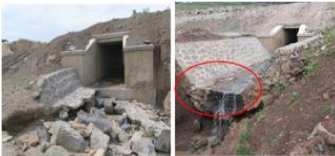
Figure 1: Outlet Scour of culvert (site report, 2013)
