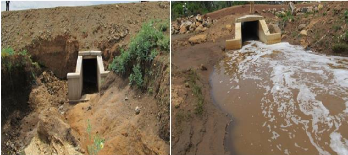
Figure 2: Inlet scours and ponding (Ethiopian Railway Corporation, site report 2013)
