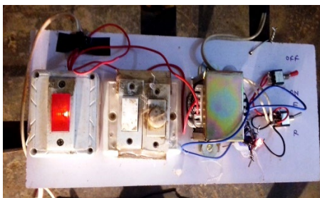
Figure 4: Control panel systems
