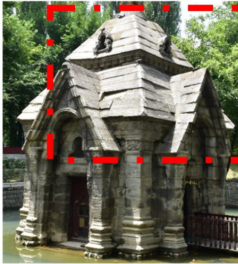
Figure 12 Shikhara of Pandrethan Temple, One of the Best Preserved Shikhara in Kashmiri style (in Red) of Temple Architecture
